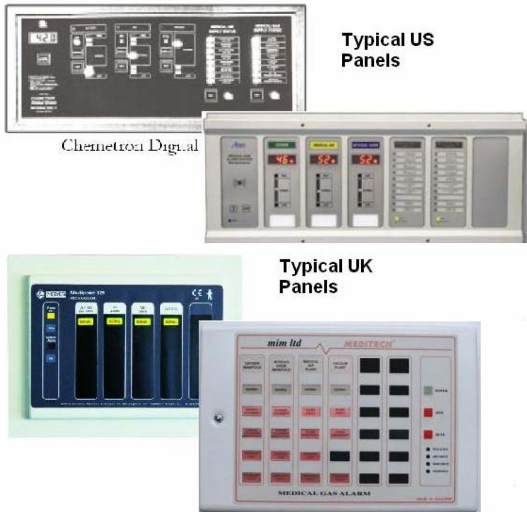
Figure 22: Typical Medical Gas Plant alarm Panels from US and UK.
