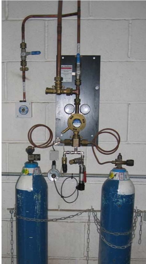
Figure 26: Entonox emergency manifold.
