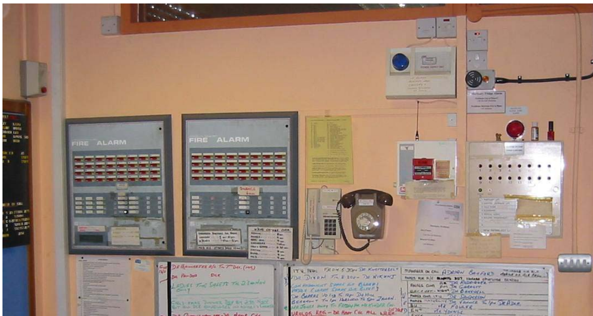
Figure 2: Seven of 18 single-vendor alarm systems interfaces in a control room.
