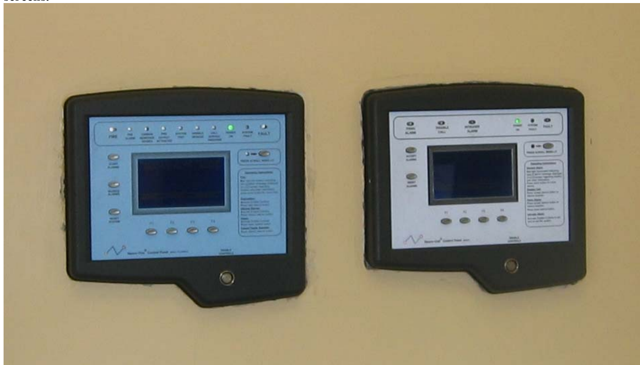
Figure 10: Picture showing integrated alarm system interfaces. Seven once separate systems are accessed and monitored from these screens.
