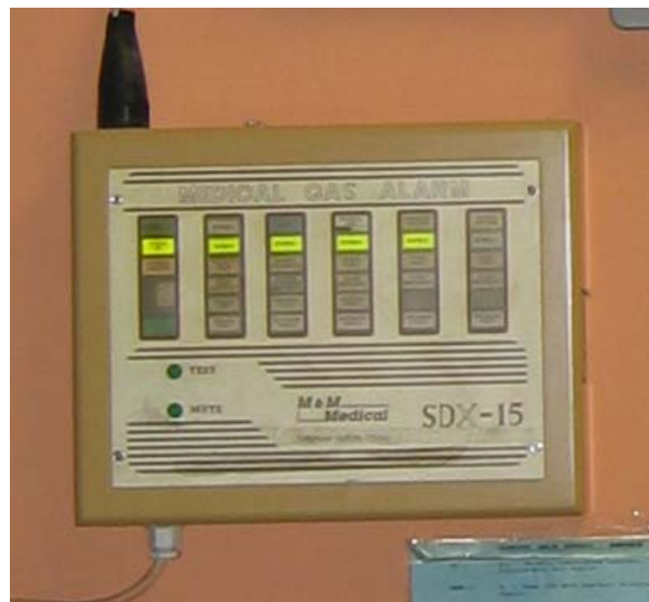
Figure 3: Single vendor medical gas alarm system interface-
