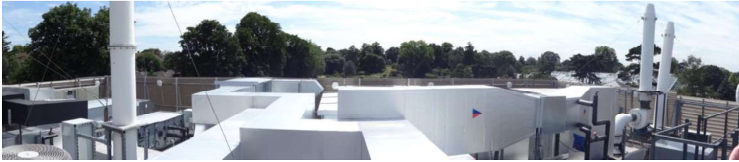
Kew Gardens roof plant space on the science teaching building- a very congested area due to many duct exhausts from fume cupboards
